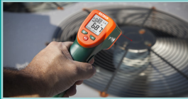
Test for temperature in HVAC systems
